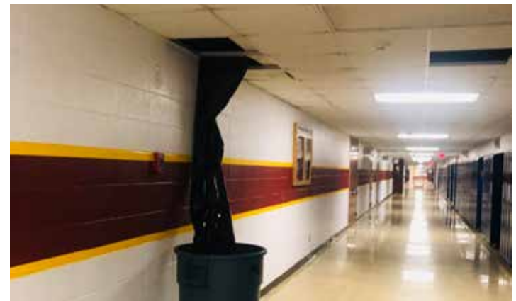
The school "fixes" the leaks coming from the ceiling with trash bags and cans.
